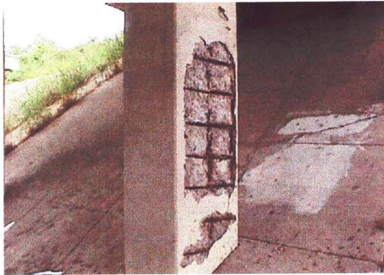
SPALL/REBAR IN COLUMN "B", BENT #3
